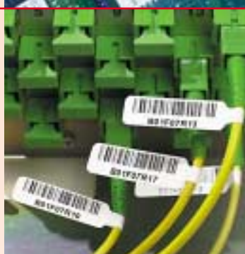
Data communications equipment labels
