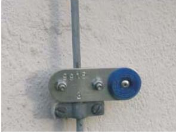
Lightning Protection Maintenance
