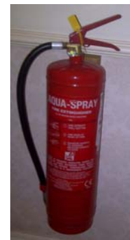
Fire Extinguisher Inspection
